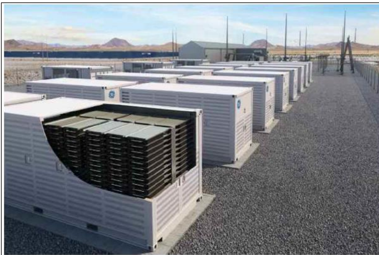
Figure 5: Typical BESS Arrangement
